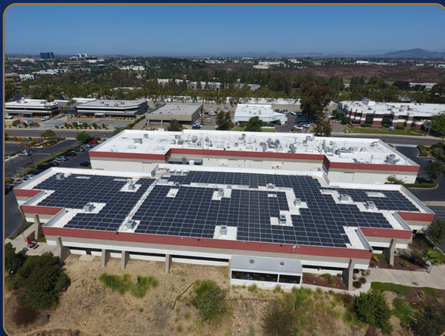
COMMERCIAL ROOFTOP SOLAR ARRAY • SOLAR GAIN INSTALLATION
