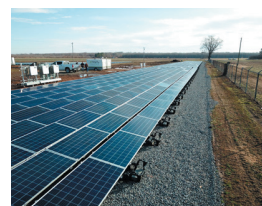
Brinkley Water Treatment Plant 600 kW
